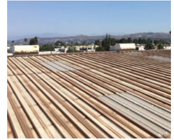
Rusted metal roof
