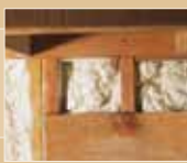
SELF-ADHESIVE SPRAY SEALS SMALL, TIGHT SPACES IN THE UNDERSIDES OF ROOF SHEATHING AND FLOOR BOARDS.
